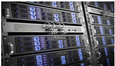
Secured data server - UMCU
